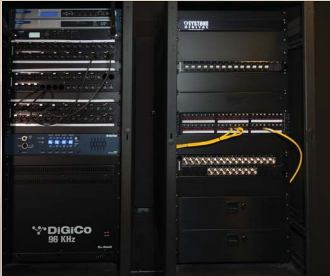
All of the signals from the stage collect at the stage rack. Then lines are distributed between the stage rack and the control booth rack for patching.
